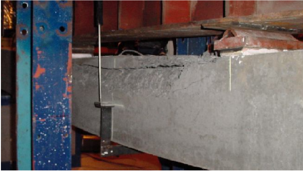
Figure 10. Concrete cover spalling off
